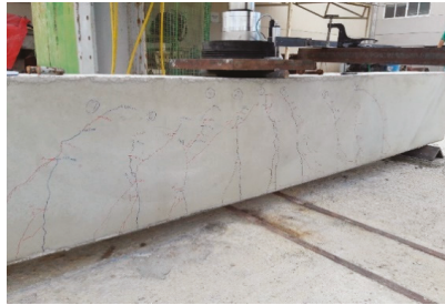
Figure 21. Visual control of cracking in the 300 × 500 mm beam.
