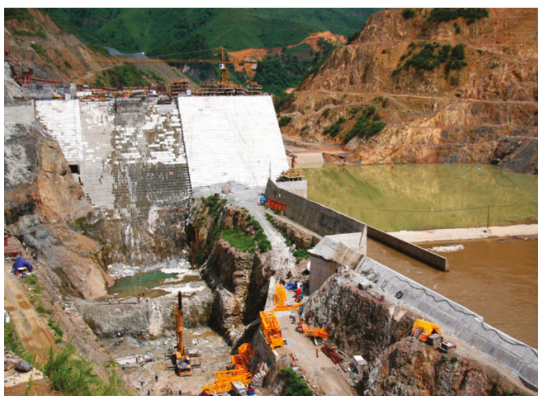
Figure 1. Ban Chat hydroelectric plant in Vietnam [6].
