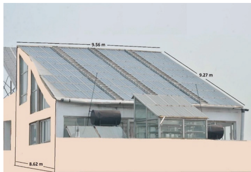
Figure 5. BAPV/T system installed at Sodha BERS complex, Varanasi (25.33° N, 82.99° E) [134].
