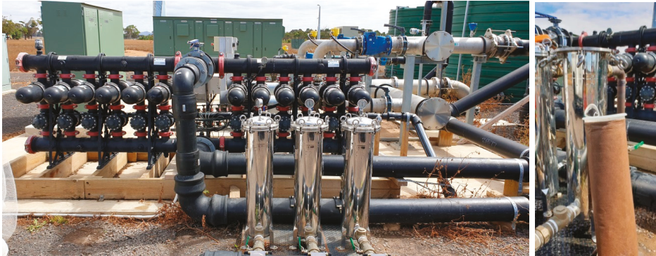
Figure 8. (Left): Central manifold ASR System with temporary prefiltration unit that includes a 20 \mu\text{m} spin Klin disc (the 12 black cylinders) followed by a 1 \mu\text{m} bag filter (the 3 upright cylinders). (Right): clogging of the 1 \mu\text{m} bag filter after \sim 2 days of operation.
