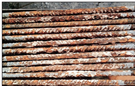
Figure 3. Rebars after the first treatment according to standard ASTM G1-03 (2017) [39].
