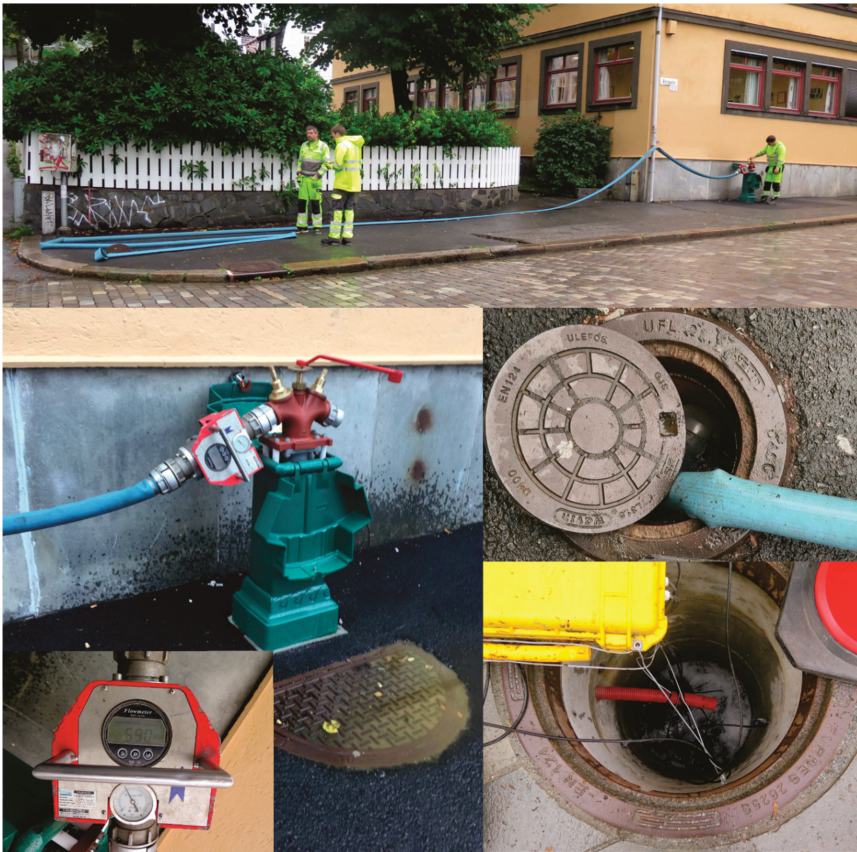
Figure 7. A fire hydrant served as a water source, providing ca. 600 L water per minute.
