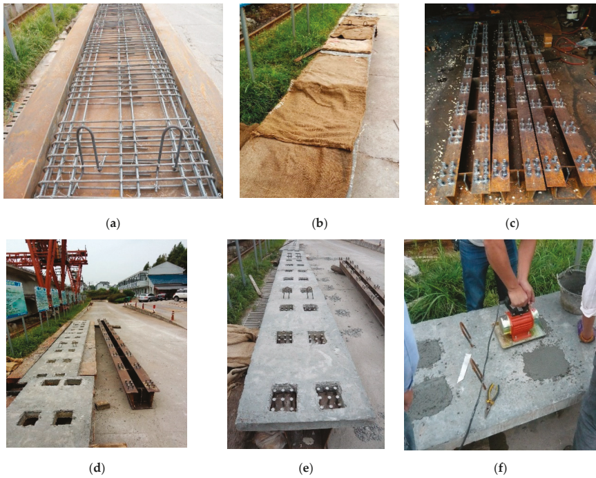
Figure 2. Fabrication process of the experimental beams: (a) formwork erection and reinforcing case binding; (b) casting and curing of concrete slab; (c) stud welding of test specimens; (d) completion of the concrete slab and steel U-type girder; (e) placing of concrete slab on steel box girder to make it composite; (f) reserve hole filling.
