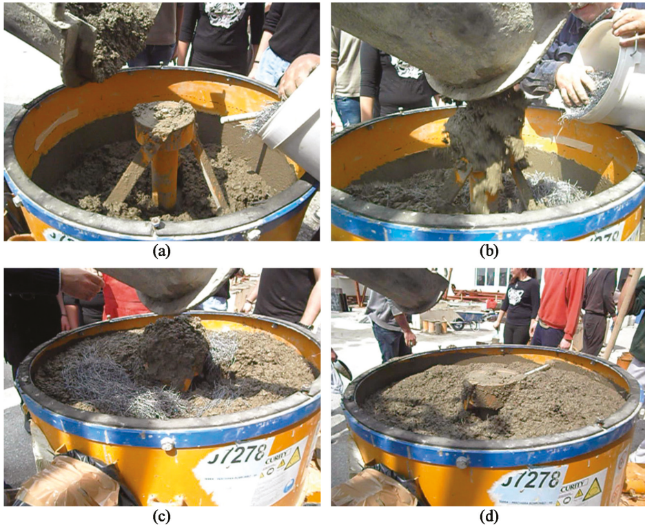
Figure 1. Preparation stages of steel fiber reinforced concrete: (a) Pouring of ready-mix concrete gradually into the pan type mixer; (b) and (c) gradual addition of the steel fibers into the fresh concrete mixture during stirring; (d) final homogeneous wet steel fiber reinforced concrete mixture.
