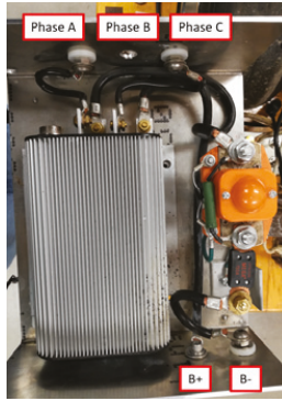
Figure 2. DC/AC inverter used in the hydraulic test bench.
