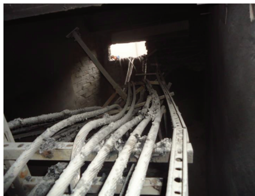
Figure 1. A destroyed cable supply system [16].
