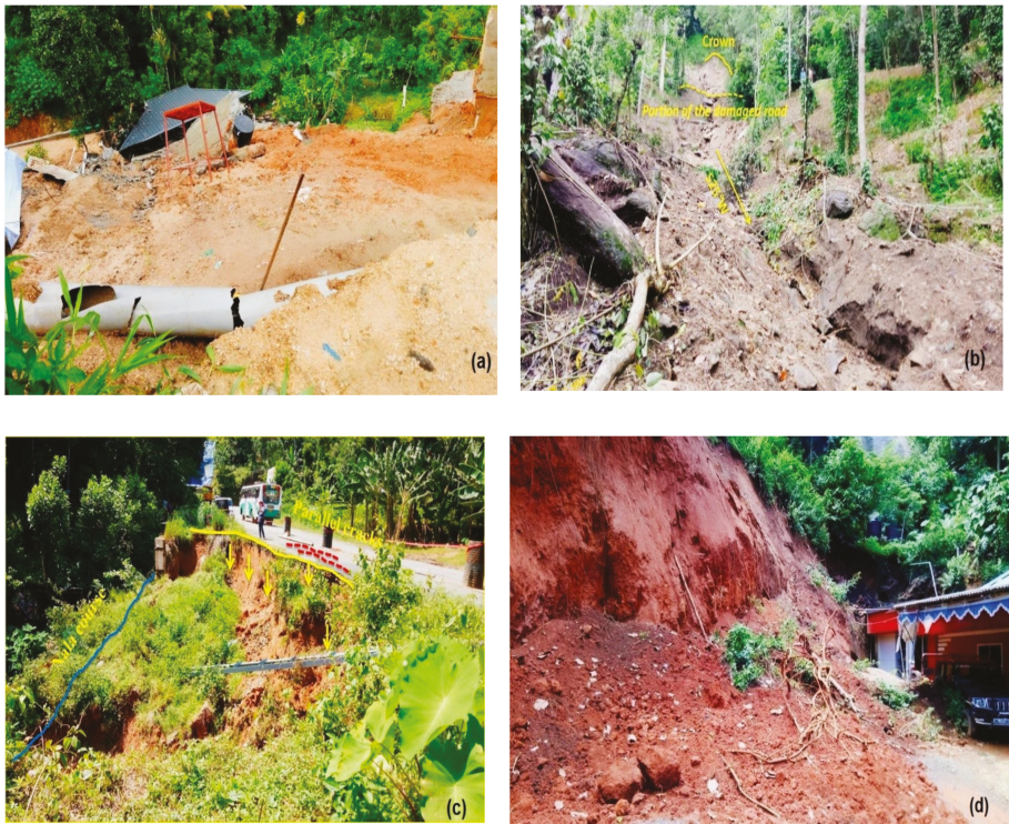
Figure 2. Damages that happened due to landslides in the Idukki district in 2018. (a) Debris slide at Anachal. (b) Debris flow at Kallimai. (c) Subsidence at Kallarkutty approach road. (d) Earth slide at Cheruthoni [22].
