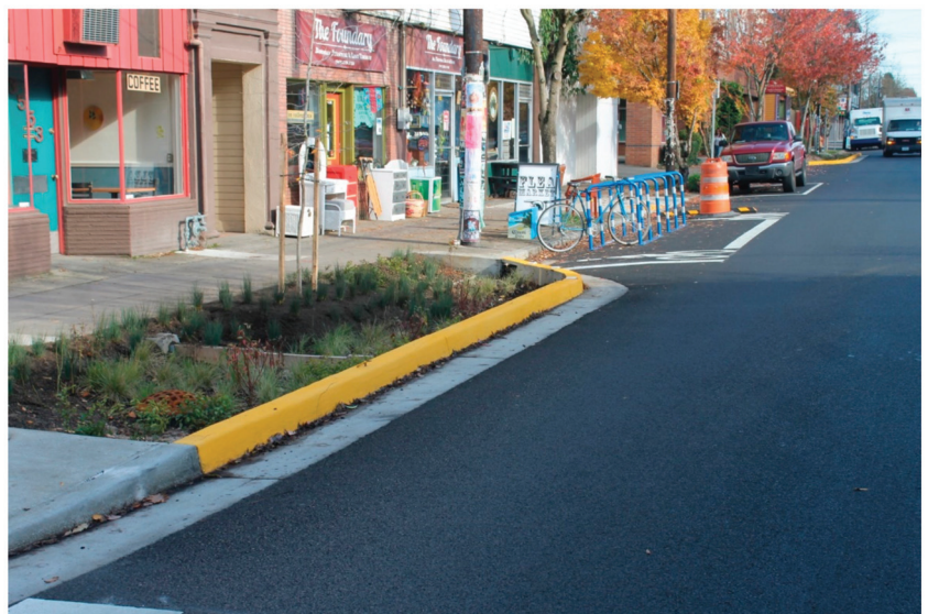
Figure 2. Curb extension in Portland (OR) to catch runoff from the roadway and the sidewalk.
