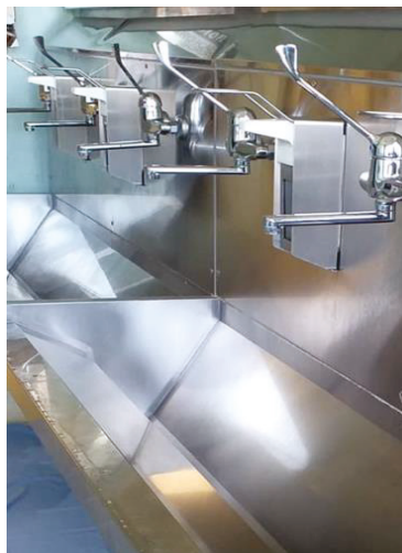
Figure 4. SHWOs with elbow-operated manual faucets without TMVs.
