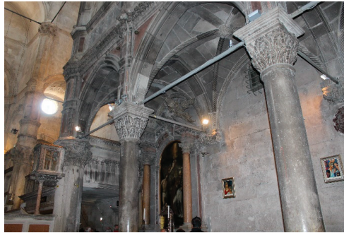
Figure 1. Cathedral of St. James in Šibenik (Croatia). Tie rods are supporting the walls and arches.
