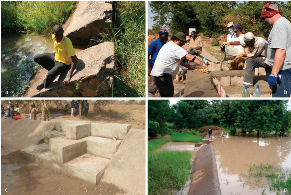
Figure 7. The rebuilding process in Kofeba: (a) the old barrage ; (b) the building phase; (c) the wall complete; (d) the barrage working phase (Source: Authors’).
