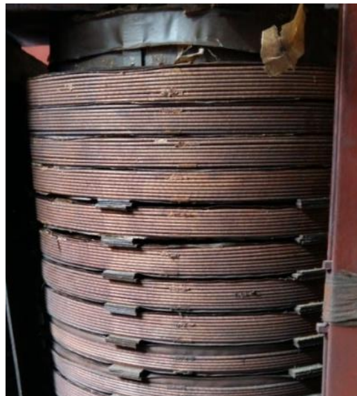
Figure 5. Example of deformation introduced into windings of a transformer: compression (reduced inter-disc distances in three gaps)—Def. 3.
