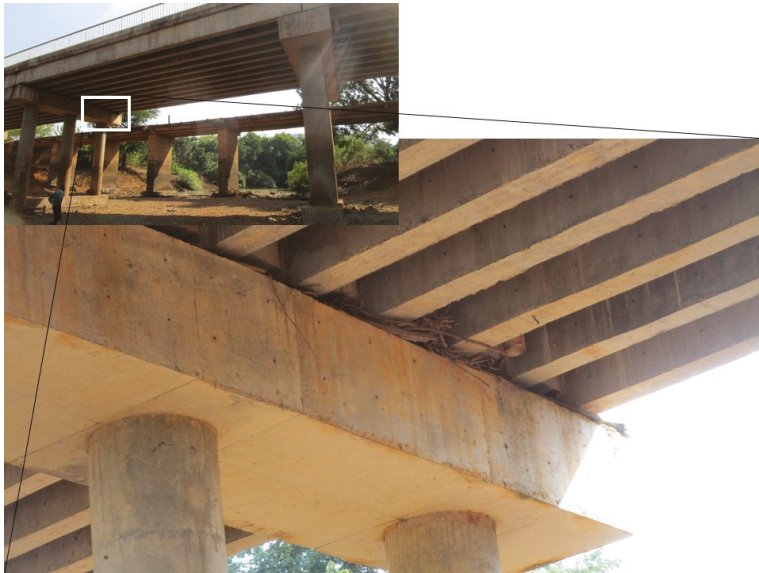
Figure 16. Pieces of branches blocked under the bridge deck of the new bridge of Komba on the Komba River (Upper Koliba/Corubal basin) after the flood of 2018. On the small picture: the new (2012) and, in the back, the ancient bridge (1950s).
