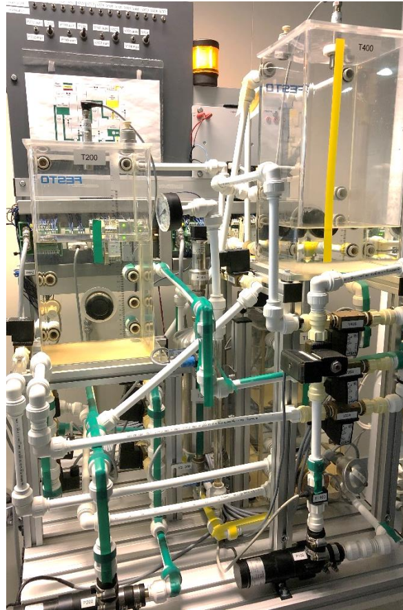
Figure 8. Aalto's water process plant.
