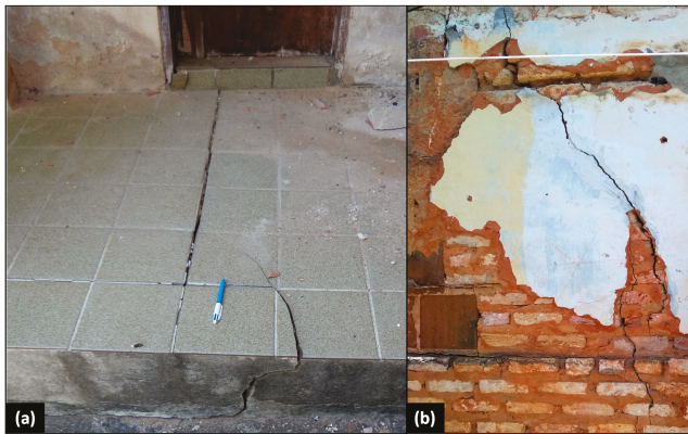
Figure 17. (a) Cracks in the floors; (b) Vertical, horizontal, and diagonal cracks in the masonry of residences in the study area.4. Discussion and Conclusions.
