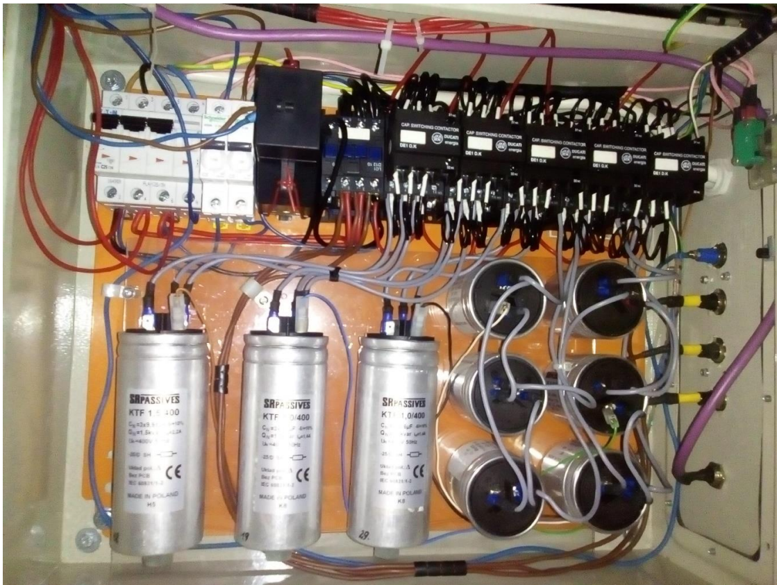
Figure 6. Capacitor battery implementation.
