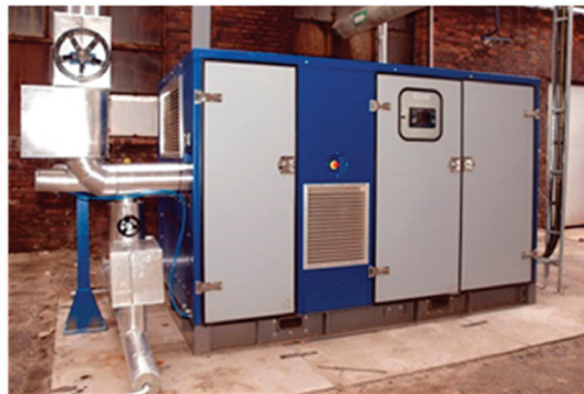
Figure 35. View of the screw expander made by Heliex Power installed at Zakłady Azotowe Kędzierzyn [164].
