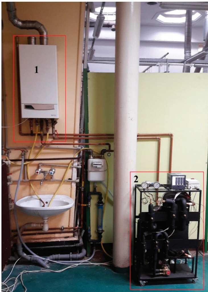
Figure 6. General view of the test-system (1—gas boiler; 2—ORC test-stand).
