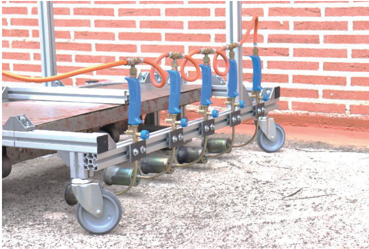
Figure 13. Individual flow regulators and parallel torches.
