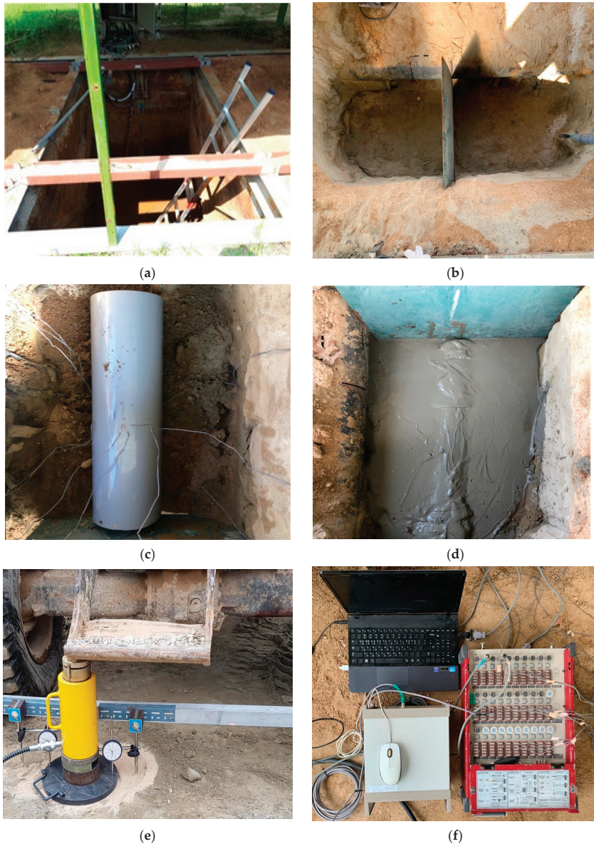
Figure 12. Plate bearing test procedure: (a) ground excavation and soil box installation; (b) ground construction; (c) buried sewage pipe; (d) CLSM construction; (e) plate bearing test; (f) test measurement.
