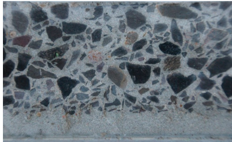
Figure 1. The structure of spun concrete in the wall thickness of a power pole.
