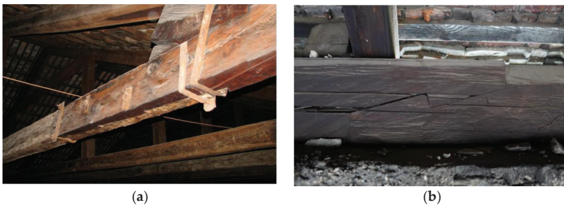
Figure 4. Examples of scarf and splice joining of wooden beams in existing buildings: (a) building in Italy, (b) building in Poland—13th century Czocho Castle in Sucha.
