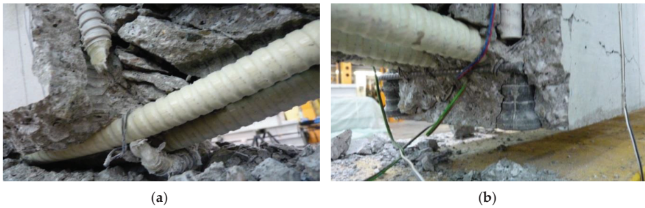
Figure 9. Failure mode of support zones: (a) reinforced with GFRP stirrups; (b) reinforced with GFRP headed bars.
