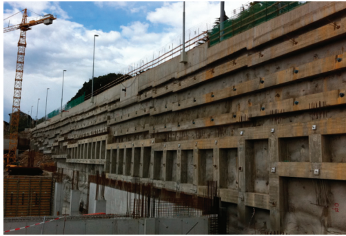
Figure 1. An example of the installed rock bolt system.
