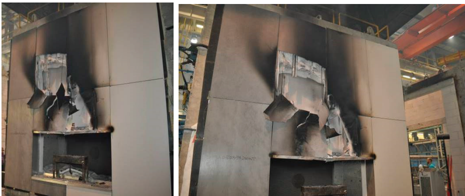
Figure 5. Ventilated facade model view after the fire source was extinguished and the test was completed.
