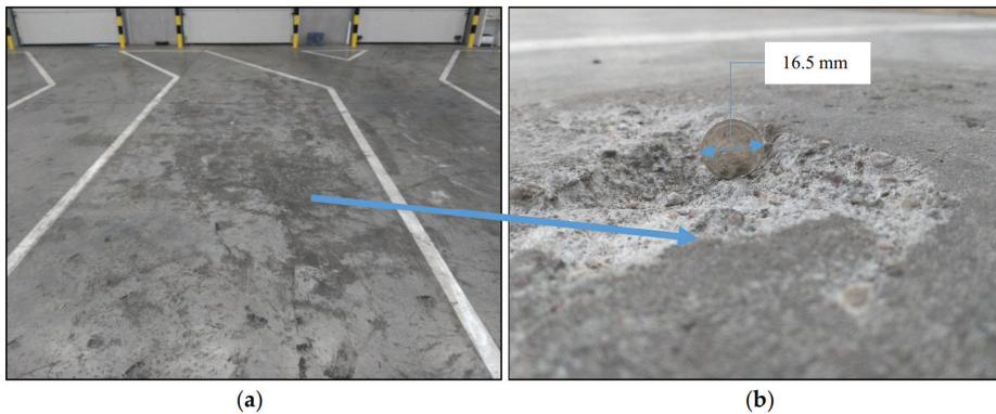
Figure 1. Example of crumbling on the top layer of concrete industrial floor: (a) General view; (b) close-up of cracked surface.
