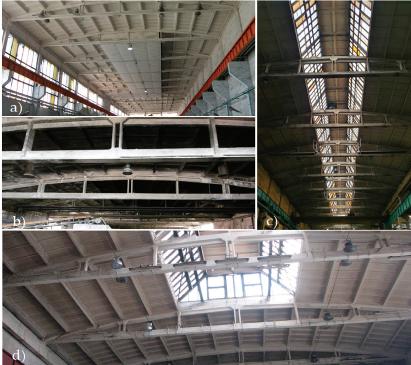
Figure 2. Factory buildings with a large number of cable post-tensioned concrete girders: (a) production and assembly hall; (b,c) production hall; (d) storage hall for powdered materials.
