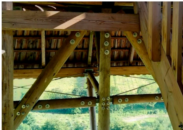
Figure 1. Practical use of connections in timber structures with mechanical fasteners and steel plates.
