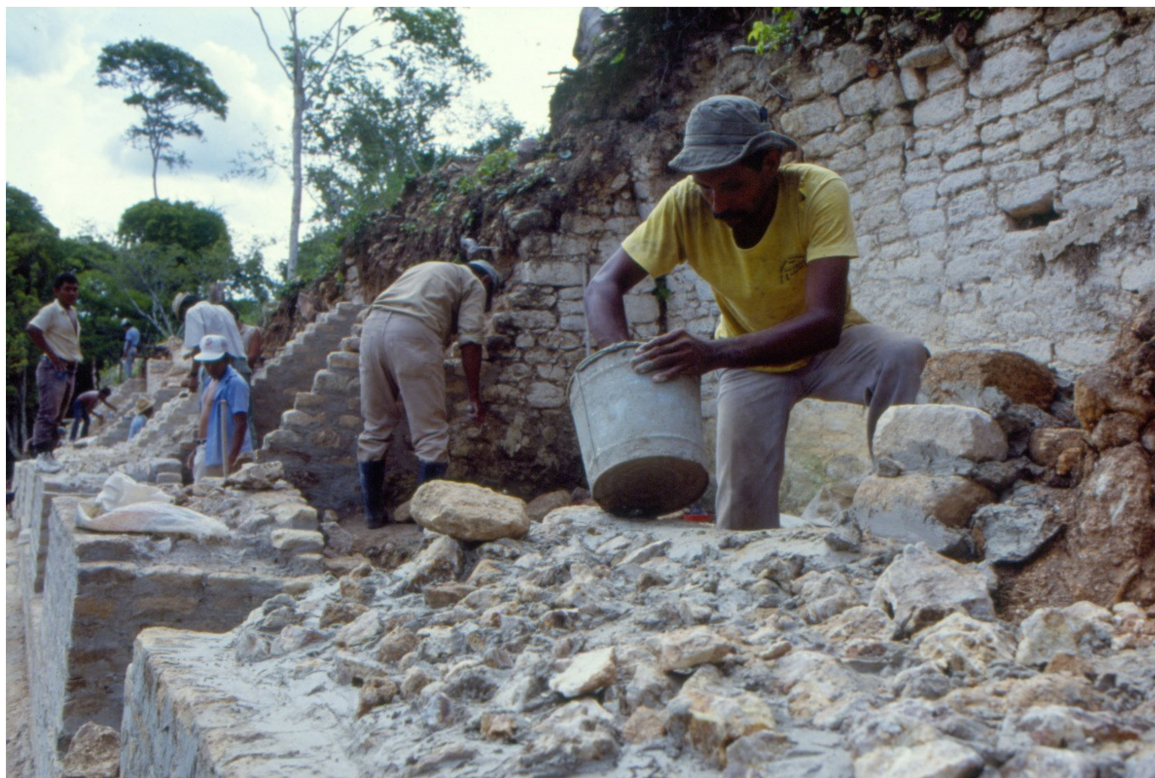
Figure 8. Stabilization being undertaken on the front face of Caana by the USAID efforts.
