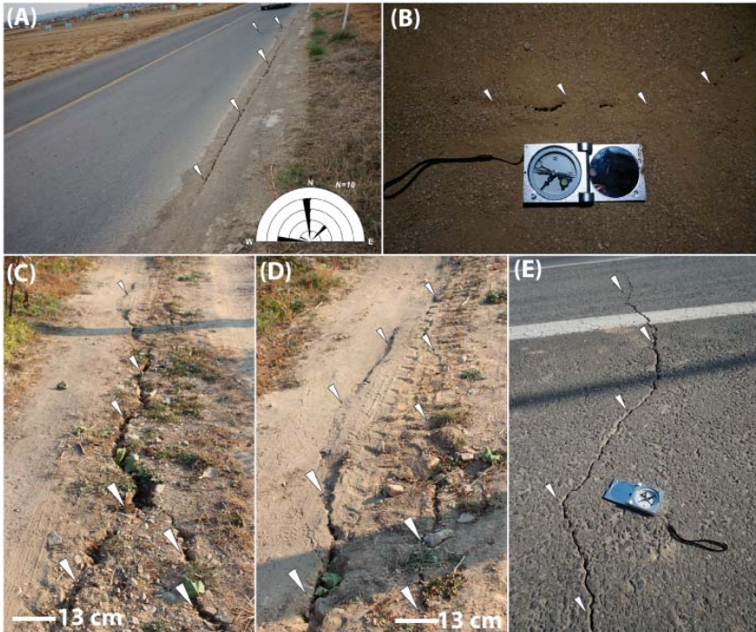
Figure 7. Field photographs showing (A) The cracks on a paved road due to differential settlement; (B–D). Ground cracks and lateral spreading along the canal embankments during the Pohang earthquake. Most of the cracks showed the N-S trend; (E) En-echelon cracks along a paved road.
