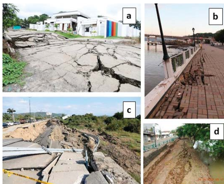
Figure 3. Example of mapped lateral spread landslides: a) deformation in alluvial plain at Jama site, the road is completely displaced for tens of meters, severe damage affected the local kindergarten ( IX_{ESI-07} ); b) deformations in river bank due to lateral spreading: soil cracks 20 cm wide at Bahía de Caráquez city ( VII_{ESI-07} ); c) total collapse of Mejía bridge at Briceño: lateral spreading, river diversion and changes of fluvial dynamics, damage on house sited on the river side ( IX_{ESI-07} ); d) lateral spreading in river bank at Calceta city: soil cracks in natural soil 20 to 25 cm wide, wavy deformations of cobbles, ( VII_{ESI-07} ); locations on Figure 2.
