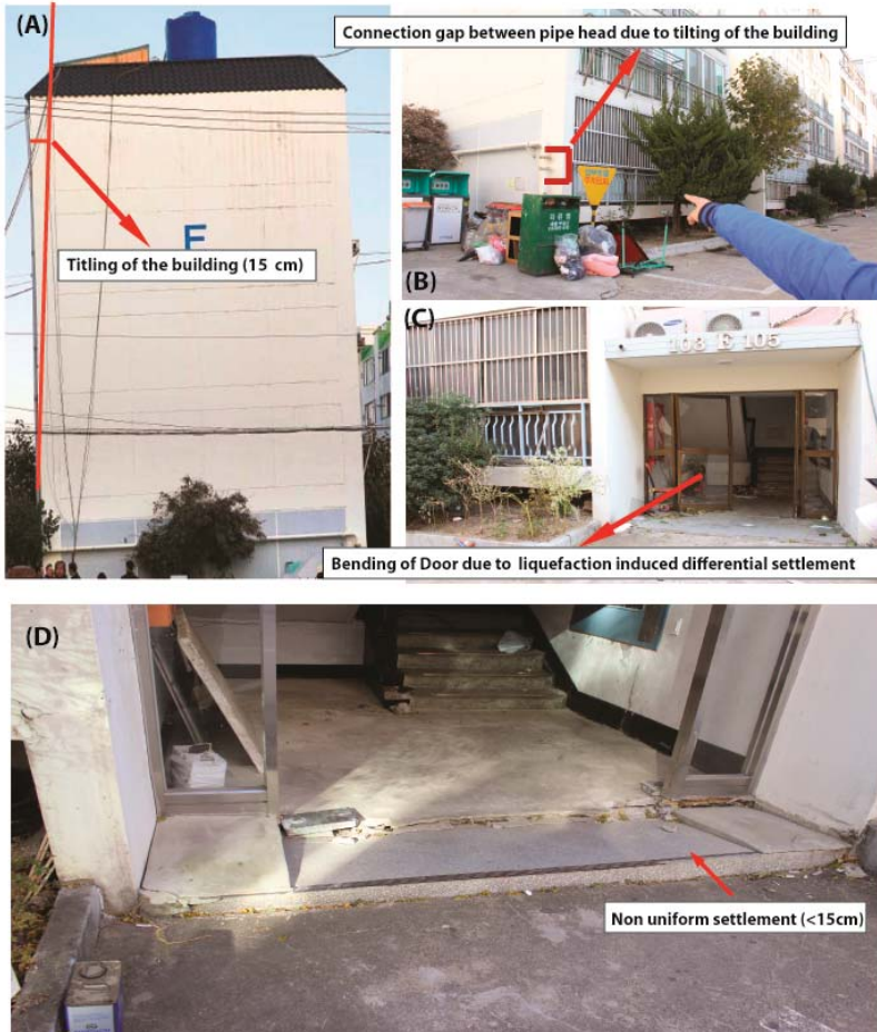
Figure 8. Photographs showing (A) a titled residential building due to differential settlement (the building was titled about 15 cm); (B) separation of water pipeline due to tilting of the building; (C,D) differential settlement observed in the basement of the residence buildings in the epicentral area (the basement of the building settled almost 15–30 cm).
