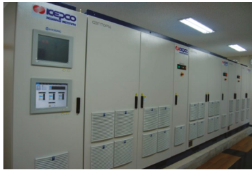
Figure 5. Grid forming inverters.
