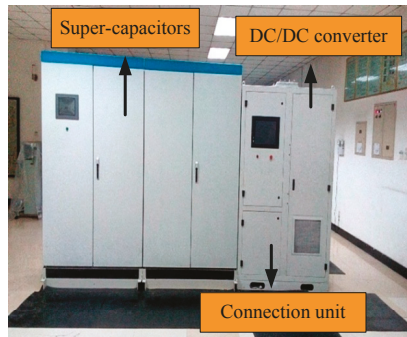
Figure 7. Super-capacitor ESS installed in traction substation.
