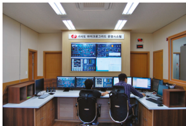
Figure 7. Energy management system.
