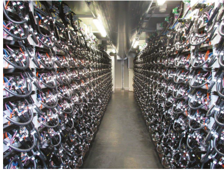
Figure 2. Racks for battery strings, installed inside an air-conditioned cabinet.
