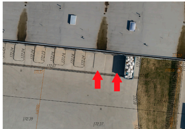
Figure 12. Visualization of the deficiencies on the vector base map using orthomosaic in AutoCAD.
