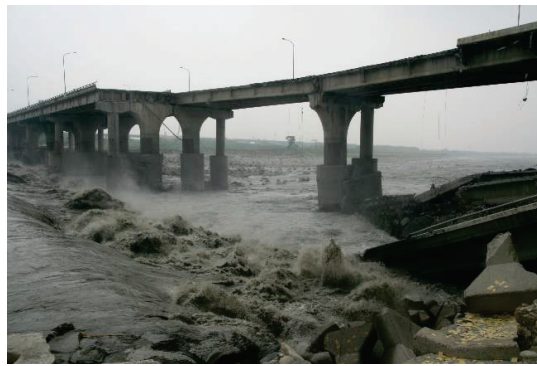
Figure 1. Failure of Houfeng Bridge in Dajia River, Taiwan due to pier-scour in September 2008 (courtesy of Yee-Meng Chiew).
