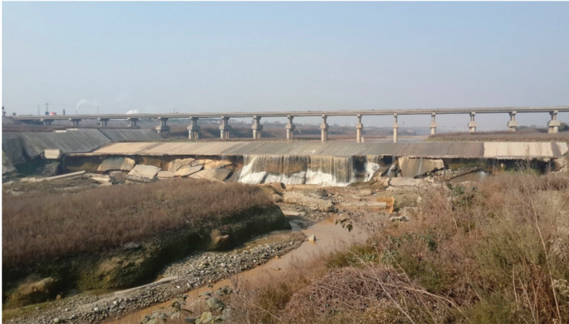
Figure 1. Scour at the grade control structure (GCS) downstream of the 105th Provincial Highway Bridge after the flood event on 9 July 2013 (discharge Q = 2710 \text{ m}^3/\text{s} ).
