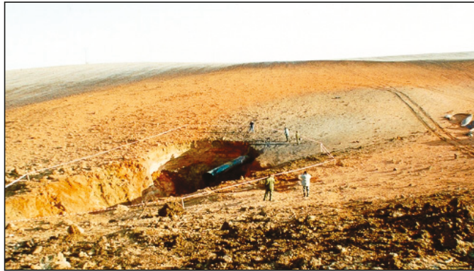
Figure 8. Gas pipeline accident due to the additional bending of a pipeline system laid on a slope with insufficient amounts of compacted subsoil.
