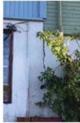
Figure 10. Crack between the buildings Strandveien 19 and 21 (NTNU).
