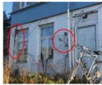
Figure 11. Humidity damage (NTNU).
