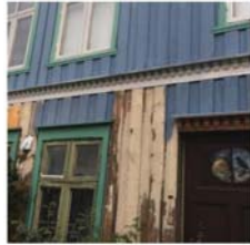
Figure 5. Deteriorating façade (NTNU).
