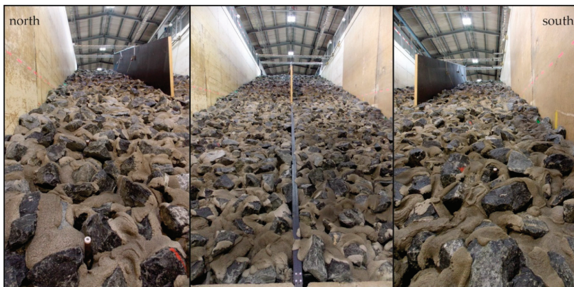
Figure 3. Partially grouted MGRRS ( v_g = 80 \text{ L/m}^2 ) in test phase one (Photos: Kreyenschulte and Kühling, 2017).
