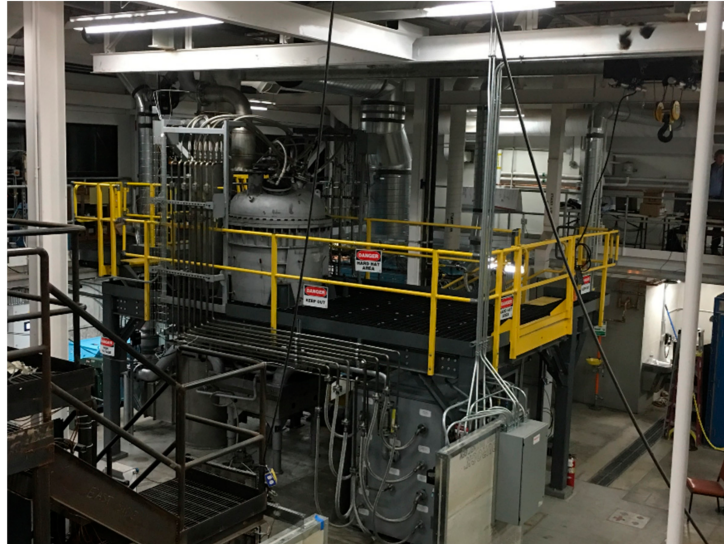
Figure 12. The Large Bench Reactor installed in the University of Utah.
