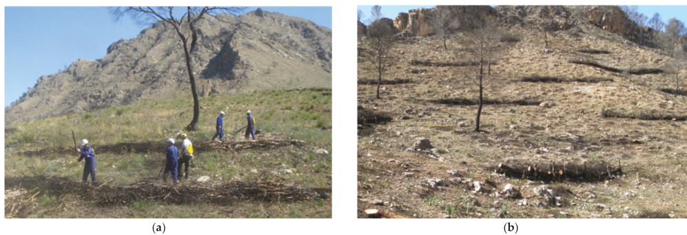
Figure 3. Photos of the construction of contour-felled log debris (a) and log erosion barriers (b) in Sierra de los Donceles forest (Castilla La Mancha, Spain).
