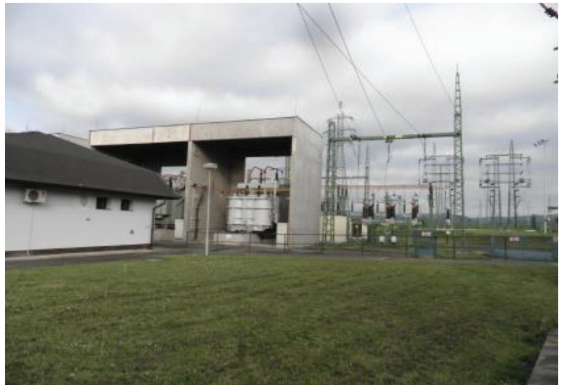
Figure 3. View of traction substation 25 kV/50 Hz.
