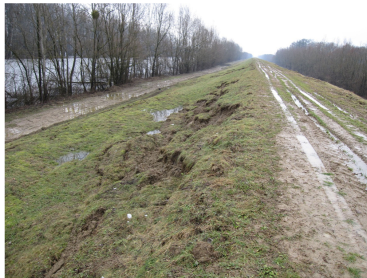
Figure 19. Dyke top structure with rutting caused by traffic and with local erosion failures typical for wet seasons.
