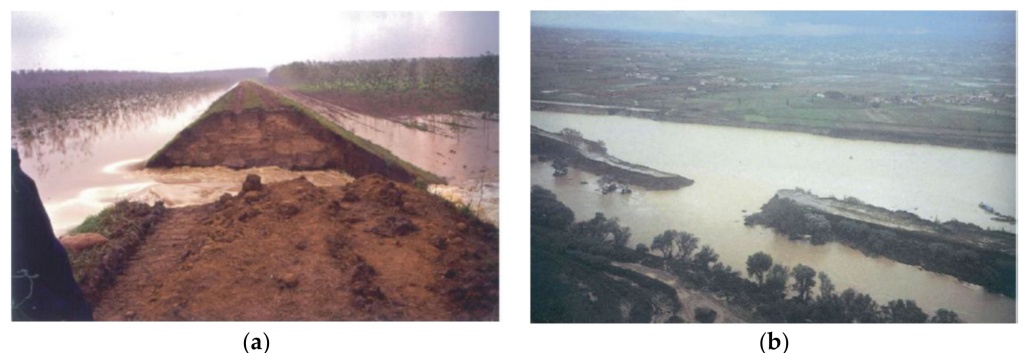
Figure 5. Examples of failure of: (a) the dyke of river Po in Mantova province (Northern Italy) during the flood event of October 2000, and (b) the dyke of river Arno in Tuscany (Italy) during the flood event of October 1992 (adapted from [17]).
