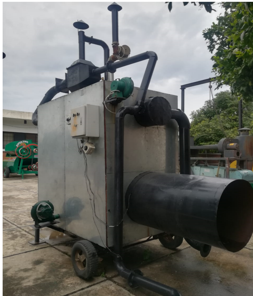
Figure 6. Side view of the modified biomass furnace.
