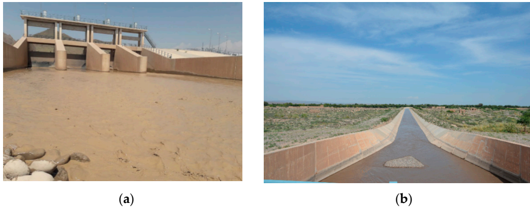
Figure 1. Sediment conditions at the diversion barrage. (a) High sediments concentration at downstream of the under sluice sections of the barrage as a result of flushing from GZ dam during 9–10 May 2019; (b) View of the main canal from canal head regulator on 10 May 2019.
