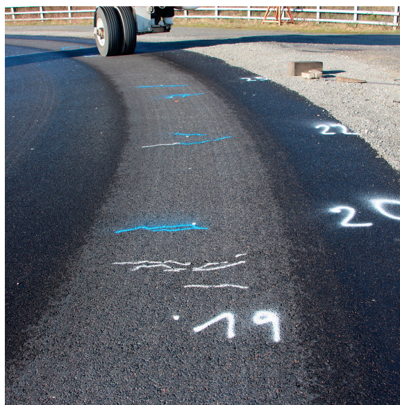
Figure 14. Surface condition of the pavement at the end of the experiment.
