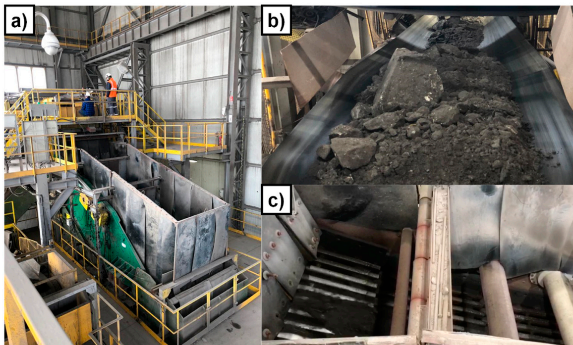
Figure 2. The investigated technical object—vibrating screen: (a) view of the whole device; (b) feed; (c) upper sieving deck.
