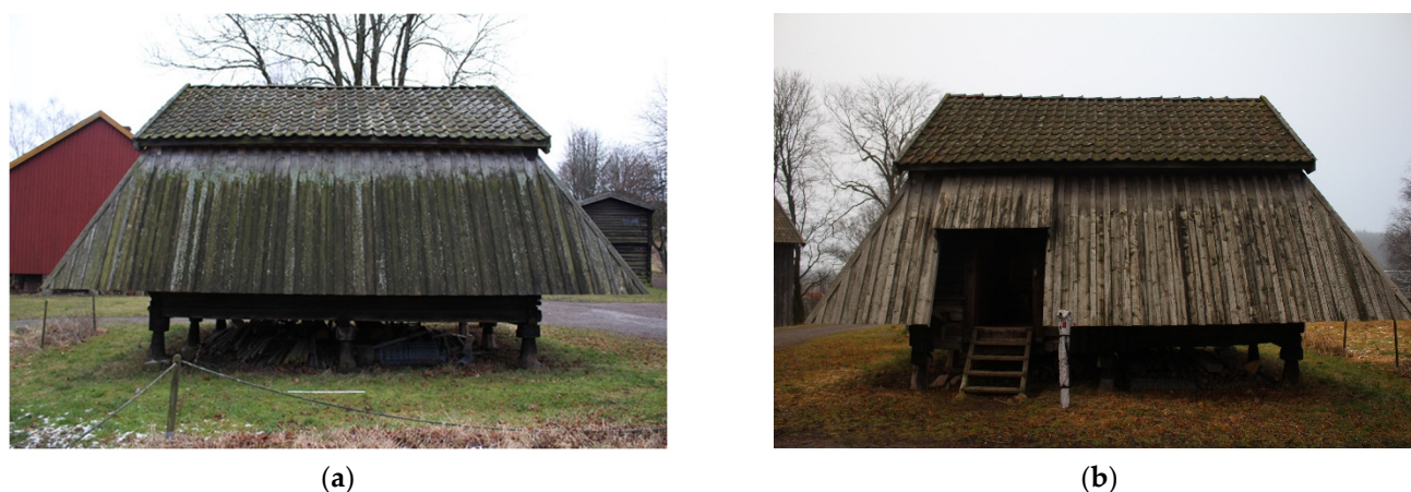
Figure 6. At the Fadum storehouse, the growth of biological organisms is more intense on (a) the north façade than on (b) the south façade.
