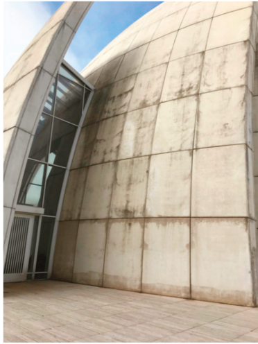
Figure 37. View of the damages on the surface of the self-cleaning concrete shells of Jubilee Church in Rome, which were caused by the local environmental dust. Reprinted with permission from [180]. Copyright©2019, Taylor & Francis Group.
