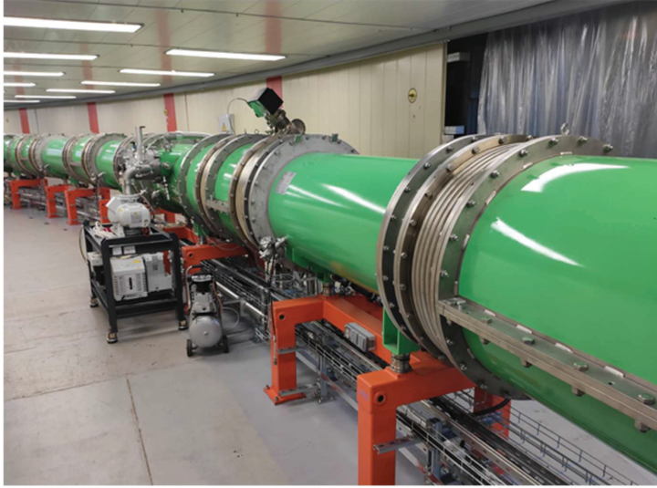
Figure 3: Booster ring system based on superconducting magnet technology developed at JINR Dubna for the Nuclotron accelerator. The booster is commissioned inside the iron yoke of the former synchrotron at the Veksler-Baldin Laboratory for High-Energy Physics of the JINR Dubna.
