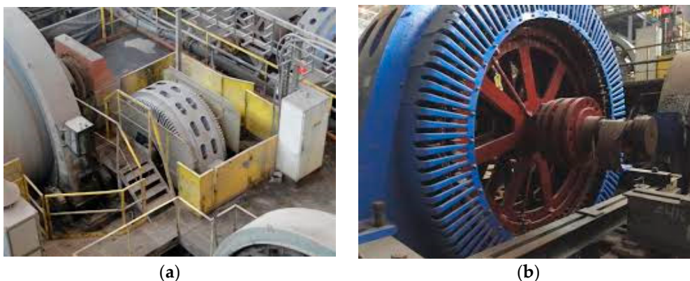
Figure 2. Ball mill drive system with low-speed SAS motor without intermediate gearbox: (a) prior to modernization, (b) after modernization on the right [34].
