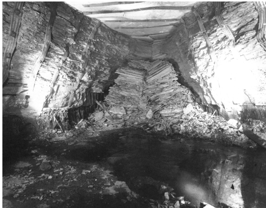
Figure 1. Collapse of immediate roof due to increased horizontal stresses in the Beckley mine [7].
