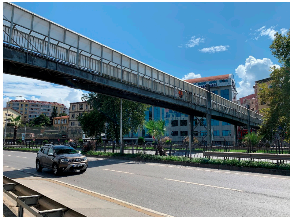
Figure 3. The view of the overpass over the road no. D010, also known as the Black Sea Coastal Highway, after construction of the roofing. Source: own study.
