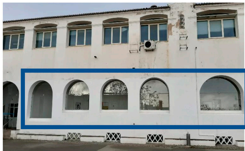
Figure 18. Floor windows 0 that will be replaced by ONYX photovoltaic windows, marked in blue.
