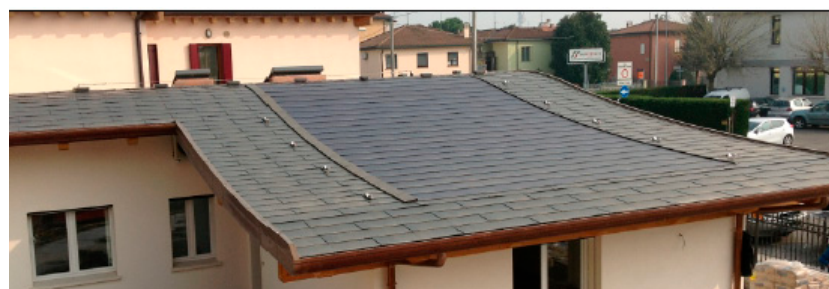
Figure 31. Tegosolar PV technology in a residential penthouse.
