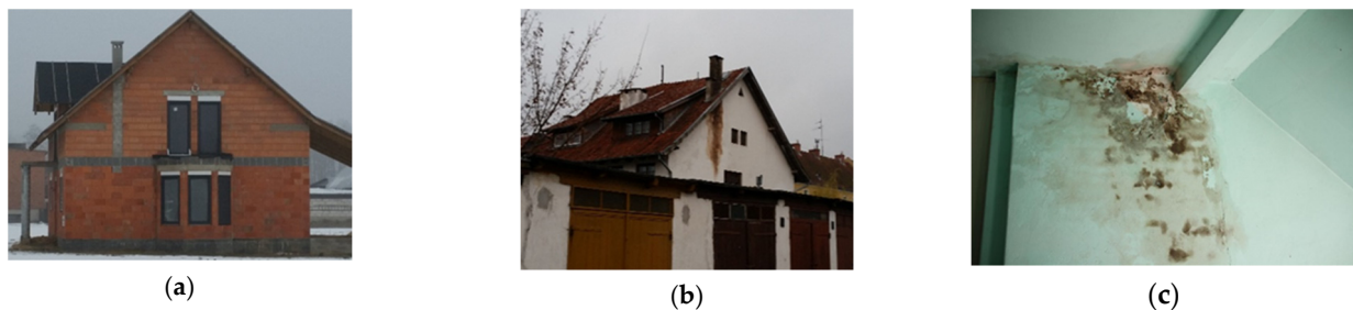
Figure 5. Consequences of inadequate protection of external and internal chimney walls (a,b) elevation, (c) inside.
