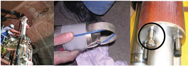
Figure 14. Pictures of distributed temperature system implementation inside vertical borehole (left). Example for a curvature guide (middle) and connector (right) to get the sensing cable through packers.
