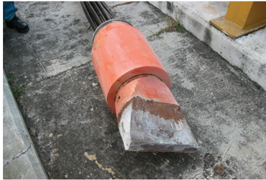
Figure 5. Failed anchoring element of cable 1 semi-harp 5 (T1S5).
