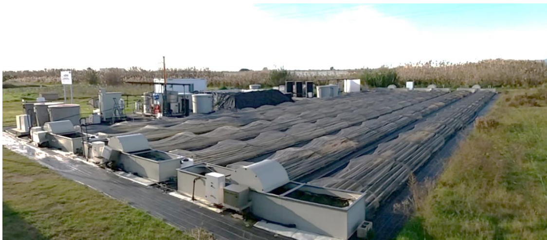
Figure 1. Global view of the demonstration-scale plant.
