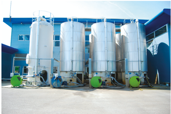
Figure 4. Tanks for artificial peloid maturation (Dax, France).
