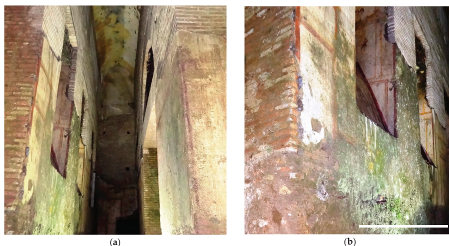
Figure 2. Two different views of the sampling site in Room 93 with the evident phototrophic biofilms causing discolouration of the walls. (a) front view of the corridor present in Room 93; (b) detailed image of the wall object of the investigation with the evident presence of the green biofilm; scale bar = 2 m.
