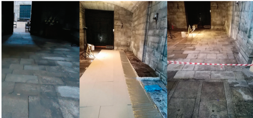
Figure 4. Detail of a church granite pavement 25 m 2 treated area following the high dimension bio-desalination optimized protocol. Area before treatment (left image), area during treatment (middle image), and area after treatment (right image).
