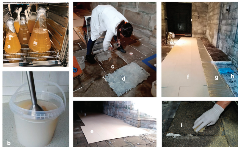
Figure 3. High dimension bio-desalination optimized protocol applied to the 233 m 2 church granite pavement. In lab preparation: (a) bacterial biomass production; (b) 2% ground agar preparation. In situ application: (c) bacterial application; (d) 2% ground agar application over the Japanese paper; (e) thermic mat applied and insulating wood panels. After treatment: removal of (f) wood panels; (g) thermic mat; (h) plastic film, ground agar, and Japanese paper; (i) final cleaning with deionized water and sponge.
